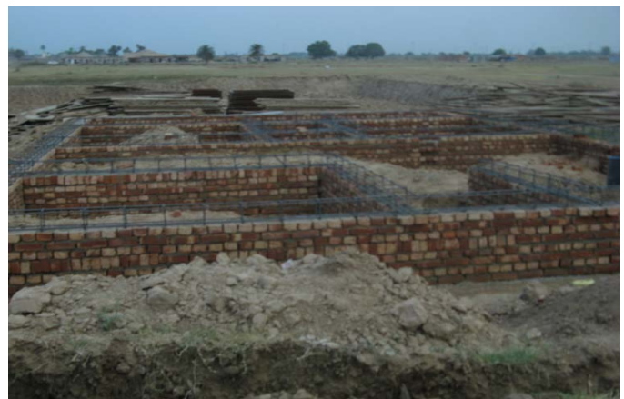
Construction in full swing on the plots handed over to the customers in Golf Links - I Mohali, Punjab
